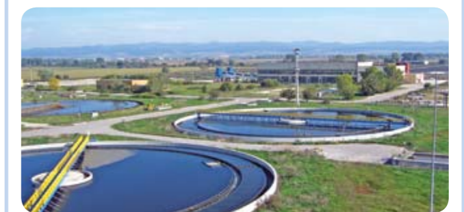
Sofia Wastewater Treatment Plant Kubratovo
